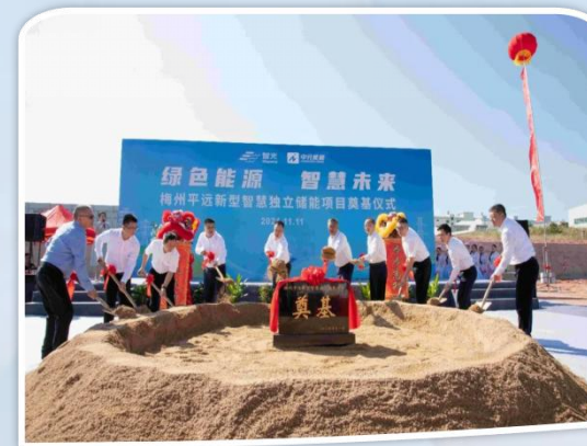
Construction starts on Phase I of the Meizhou Pingyuan Smart Energy Storage Project
